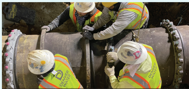
Denver Water crews install, repair & maintain more than 3,000 miles of pipelines that collect and deliver clean, safe drinking water to 1.5 million people in Denver and surrounding suburbs every day. (Photo: Denver Water)
